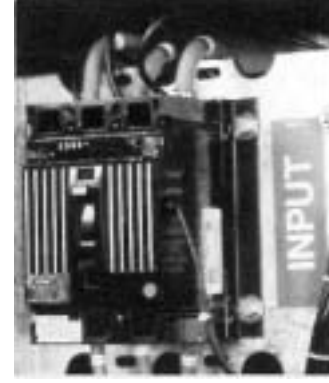
Input Circuit Breaker
